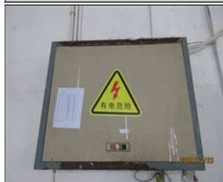
External photo(s) of the production unit(s) Switches Box Posted with Nonflammable Warning Sign.JPG
