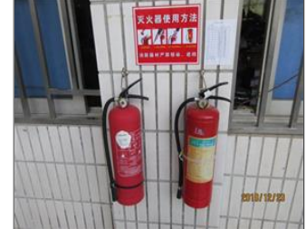
External photo(s) of the production unit(s) Fire Extinguishers.JPG
