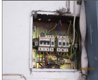
External photo(s) of the production unit(s) NC PA 7-9 7-13 Switches Box not Posted with Warning Sign or Installed with Safety Cover.JPG
