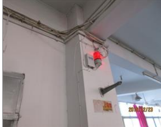
External photo(s) of the production unit(s) Fire Alarm Testing.JPG
