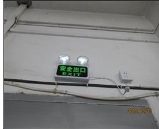
External photo(s) of the production unit(s) Emergency Lights Testing.JPG
