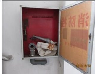
External photo(s) of the production unit(s) Fire Hydrant.JPG
