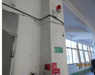
External photo(s) of the production unit(s) Fire Alarm.JPG
